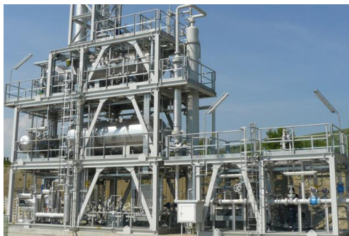
Gas Sweating Systems
