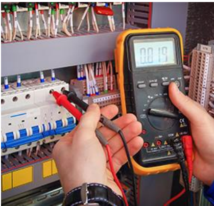
Electrical Installation, Instrumentation, And Automation Systems
