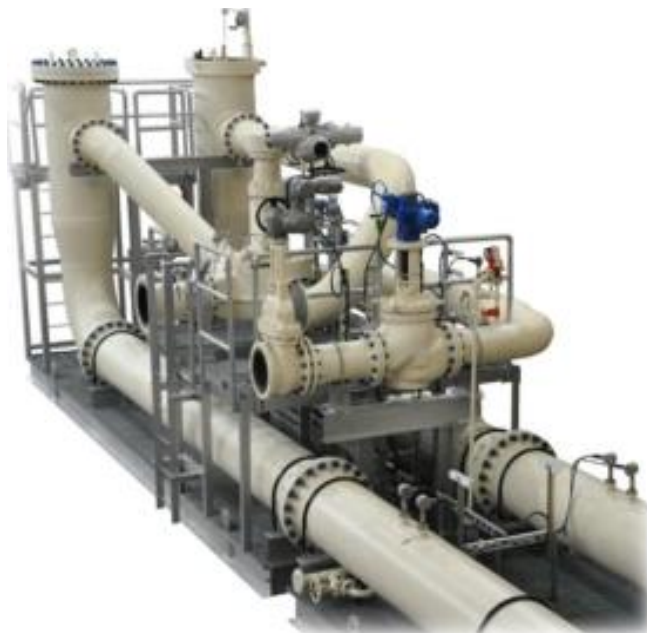
Oil&Gas Custody Transfer and Metering Station & Proving systems
