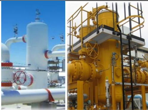
Oil /Gas /Water Filtration & Separation Units
