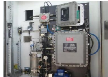
Packaged Analyzer System
