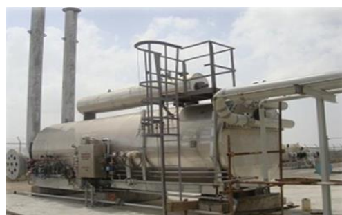
Direct And Indirect Heat Exchangers
