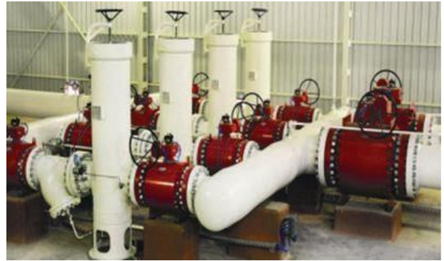
Azerbaijan 2017 12 Pcs DN500 Filter Separator
