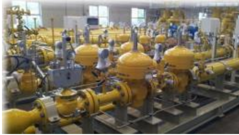
Gas Treatment and Conditioning & Regulating Systems
