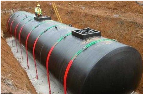
Underground Storage Tanks
